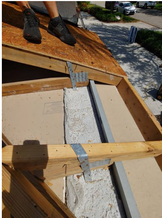
Photograph #7: Existing strap clips on the trusses have the required minimum quantity of nails on building 7861.
