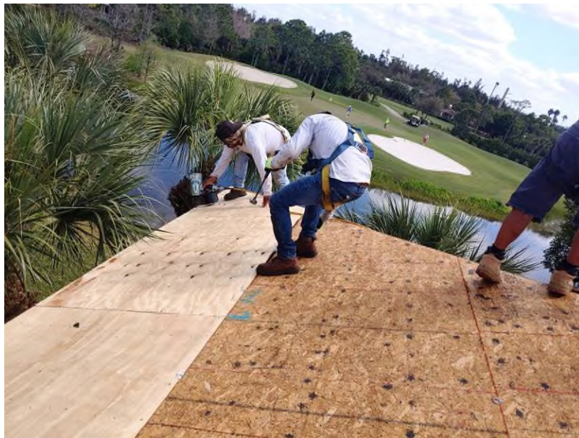
Photograph #4: Re-nail pattern at the plywood sheathing was in progress on buildings 7870.
