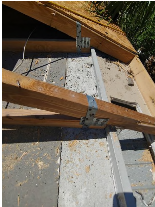
Photograph #18: Existing strap clips on the trusses have the required minimum of nails on building 21781.
