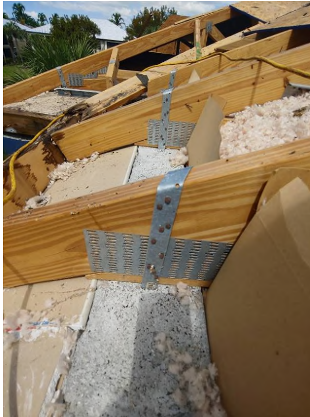
Photograph #27: Existing strap clips on the trusses have the required minimum of nails on building 21820.
