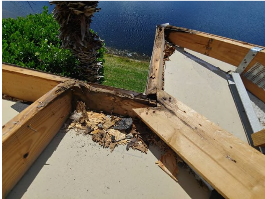
Photograph #13: Rotten fascia and truss were observed on building 21750.
