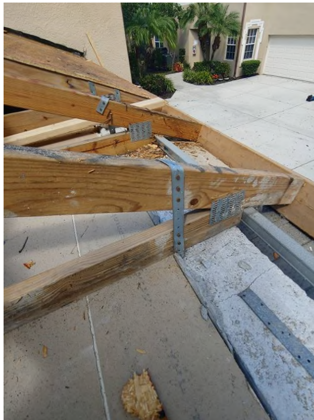
Photograph #6: Existing strap clips on the trusses have the required minimum quantity of nails on building 7861.
