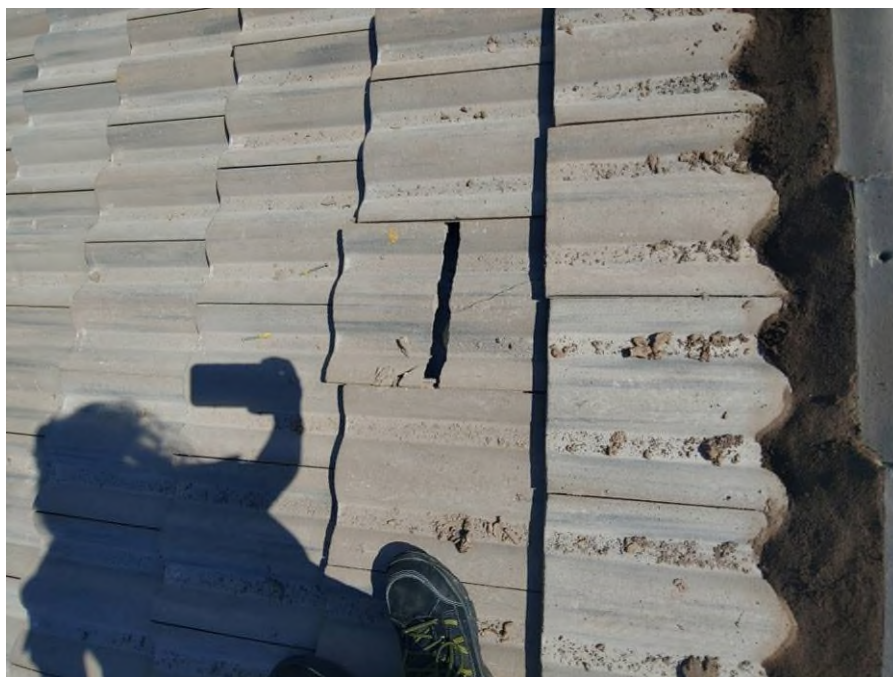
Photograph #7: Broken field tile replacement must be addressed on building 21711.
