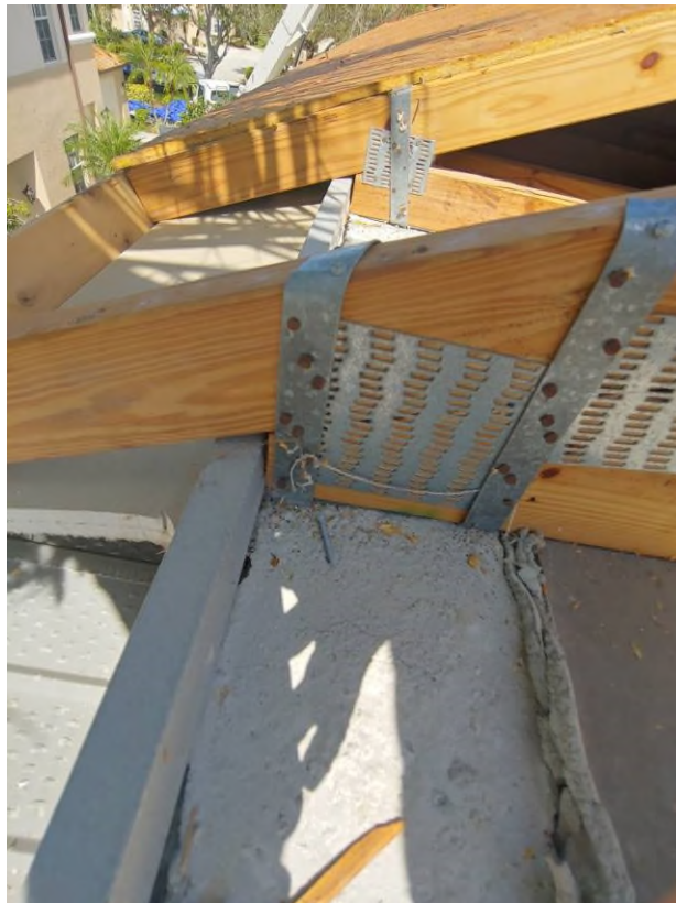
Photograph #12: Existing strap clips on the trusses have the required minimum quantity of nails on building 21750.
