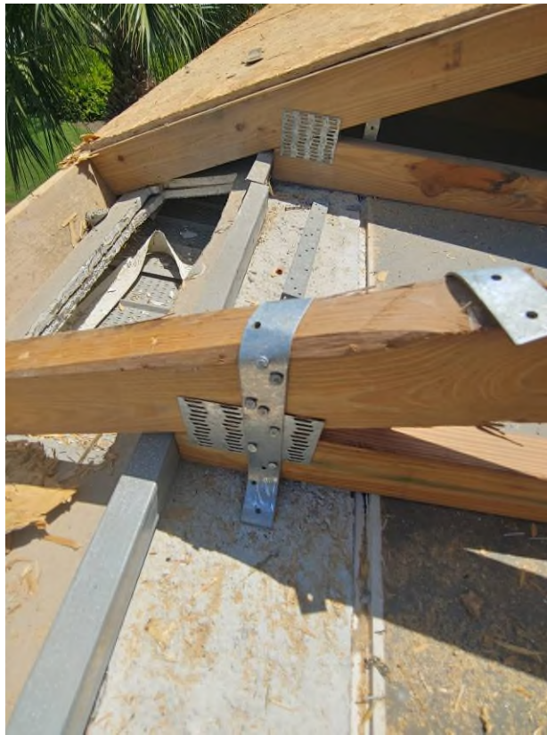
Photograph #17: Existing strap clips on the trusses have the required minimum of nails on building 21781.
