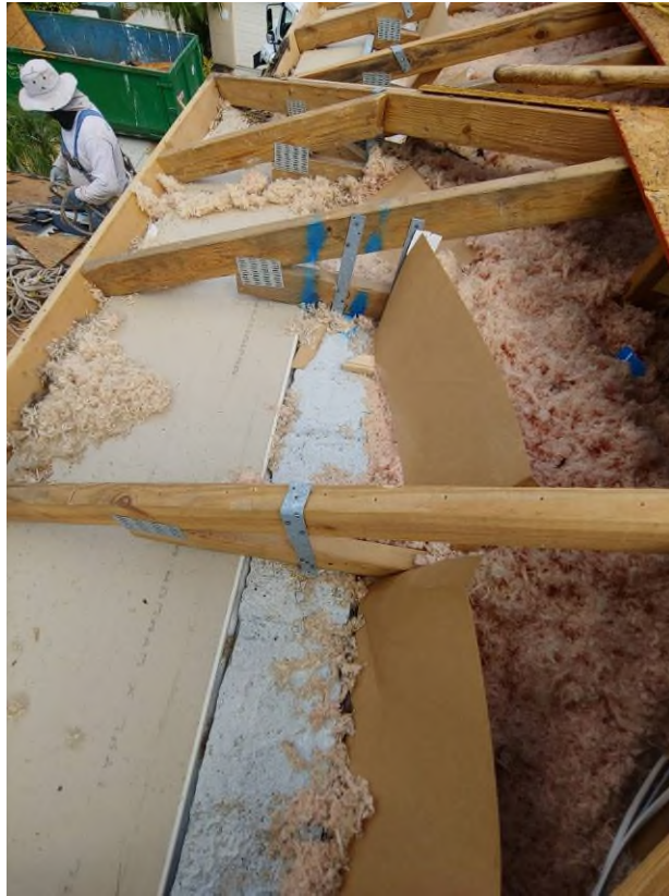
Photograph #1: Existing strap clips on the trusses have the required minimum quantity of nails on building 7870.
