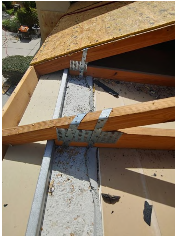
Photograph #7: Existing strap clips on the trusses have the required minimum quantity of nails on building 21740.
