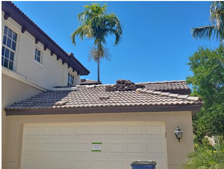
Photograph #3: Roof field, ridge and hip tile installations with polyurethane foam adhesive were in progress on building 21710.
