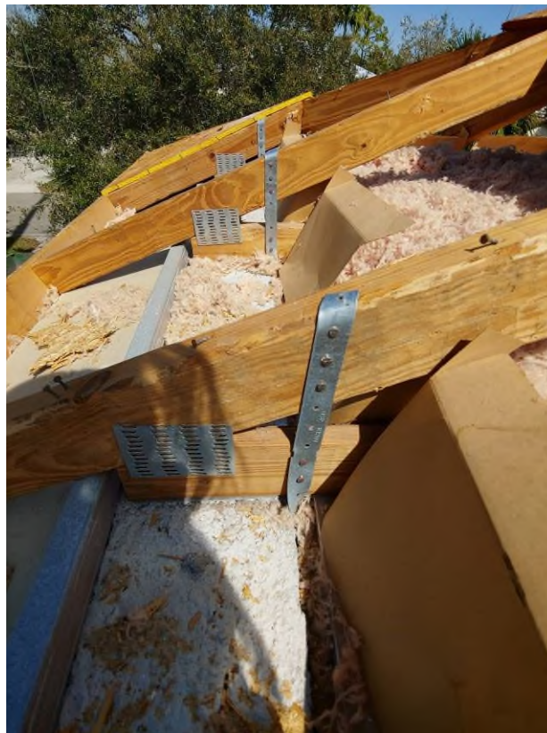
Photograph #12: Existing strap clips on the trusses have the required minimum quantity of nails on building 21740.
