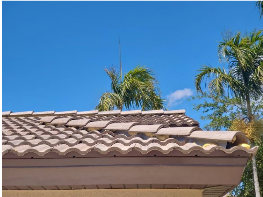
Photograph #1: Roof field, ridge and hip tile installations with polyurethane foam adhesive were in progress on building 21710.
