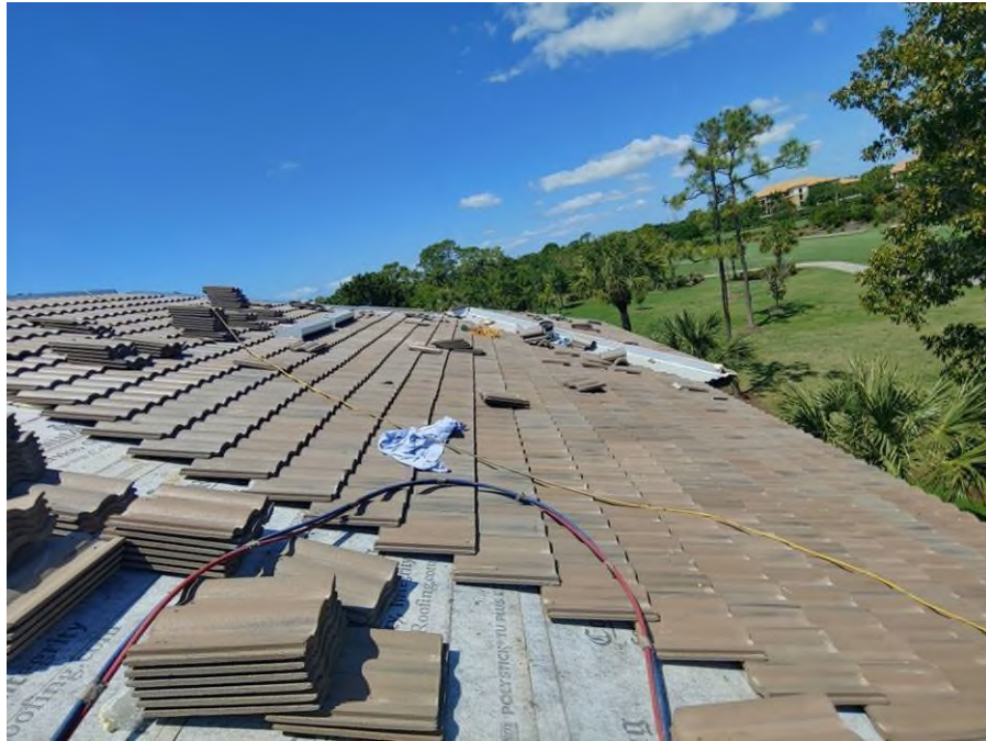
Photograph #11: Roof field, ridge and hip tile installations with polyurethane foam adhesive were in progress on building 21721.
