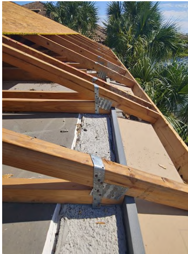
Photograph #11: Existing strap clips on the trusses have the required minimum quantity of nails on building 21740.
