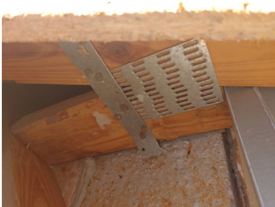
Photograph #2: Existing strap clips on the trusses have the required minimum quantity of nails on building 7870.
