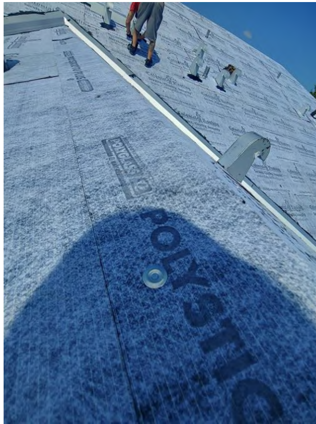
Photograph #5: Contractor must cover all exposed nails with asphalt plastic roofing cement on building 7851.
