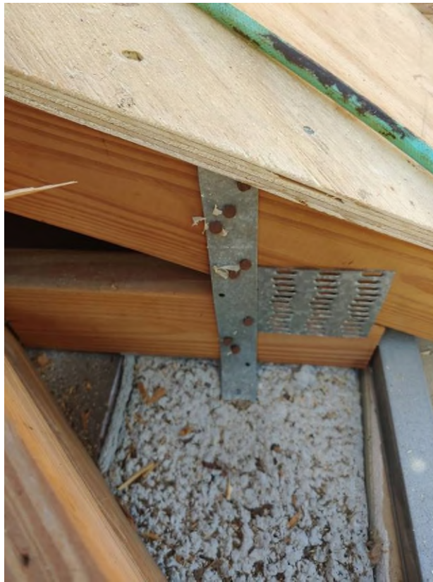
Photograph #3: Existing strap clips on trusses have the required minimum quantity of nails on building 7860.
