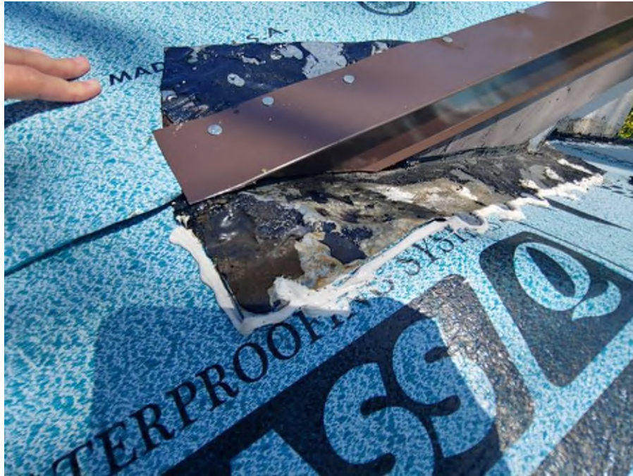
Photograph #9: Contractor must address sealant application on the metal flashing on building 7841.
