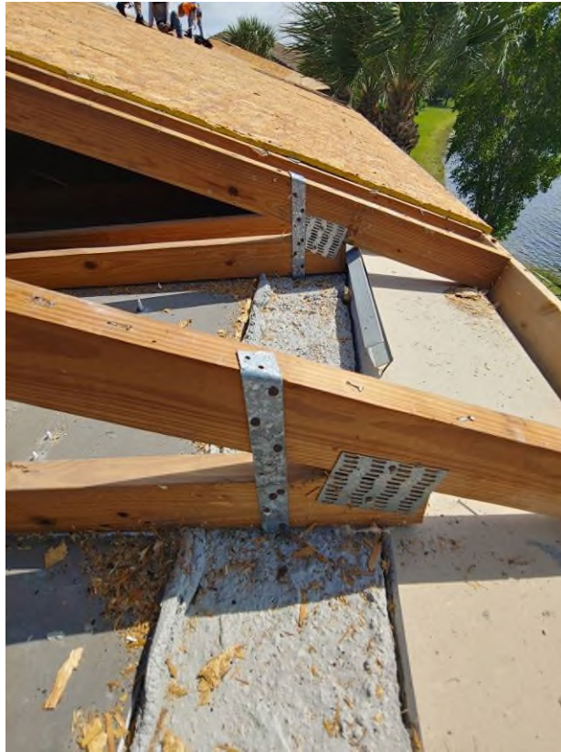
Photograph #19: Existing strap clips on trusses have the required minimum quantity of nails on building 21720.
