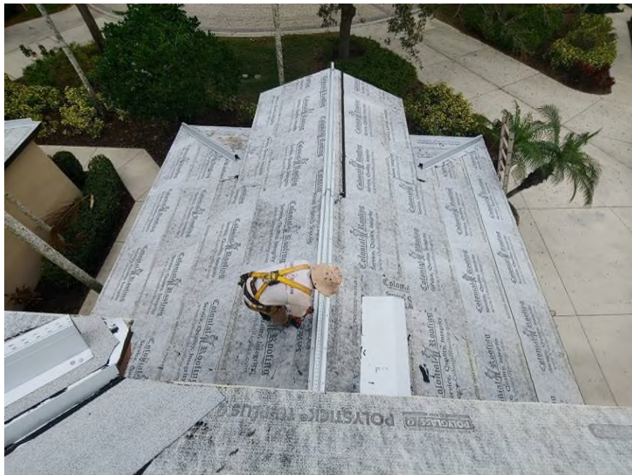
Photograph #8: V-crimp metal valley flashing, and hip/ridge metal channel installations were in progress on building 21700.
