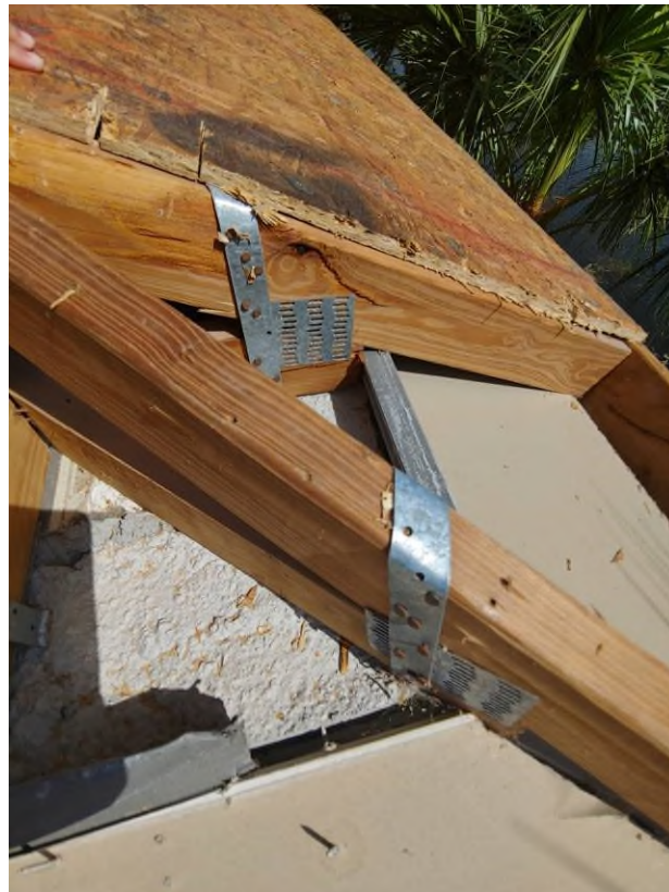
Photograph #2: Existing strap clips on trusses have the required minimum quantity of nails on building 7860.
