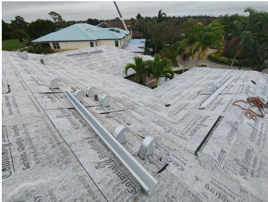
Photograph #13: V-crimp metal valley flashing, and hip/ridge metal channel installations were in progress on building 21711.
