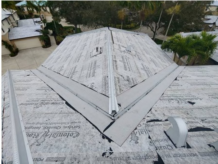
Photograph #7: V-crimp metal valley flashing, and hip/ridge metal channel installations were in progress on building 21700.
