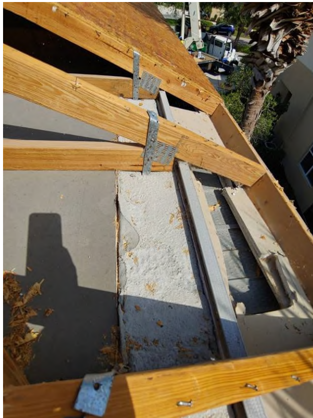
Photograph #18: Existing strap clips on trusses have the required minimum quantity of nails on building 21720.
