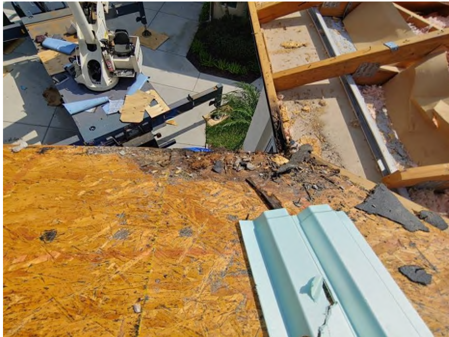
Photograph #20: Rotten plywood sheathing was observed on building 21720.
