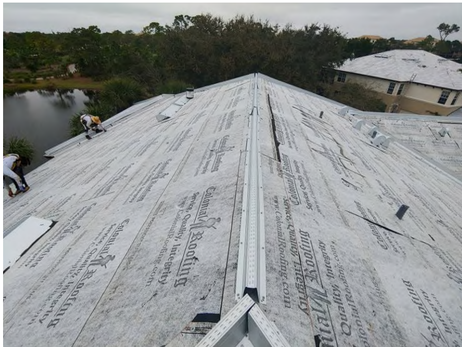
Photograph #6: V-crimp metal valley flashing, and hip/ridge metal channel installations were in progress on building 21700.
