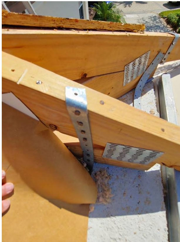
Photograph #3: Existing strap clips on trusses have the required minimum quantity of nails on building 7851.
