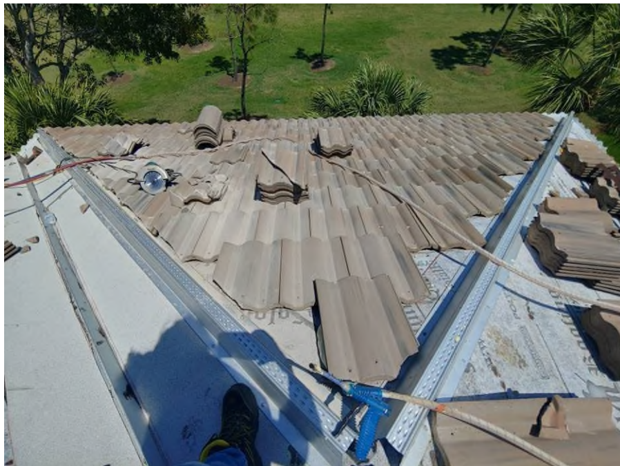
Photograph #10: Roof field, ridge and hip tile installations with polyurethane foam adhesive were in progress on building 21721.
