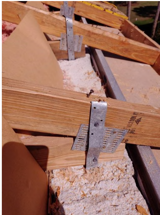
Photograph #7: KEG observed a lack of nails on a few existing straps on building 21721. N8d nails were installed during the site visit to comply with the Florida Building Code.
