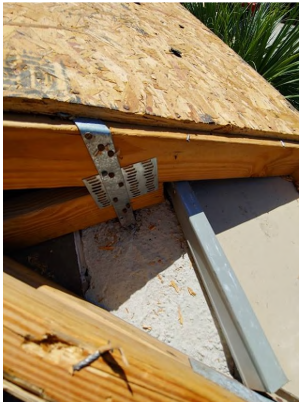
Photograph #4: Existing strap clips on trusses have the required minimum quantity of nails on building 7851.
