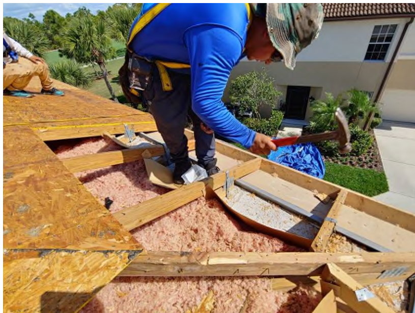
Photograph #8: KEG observed a lack of nails on a few existing straps on building 21721. N8d nails were installed during the site visit to comply with the Florida Building Code.
