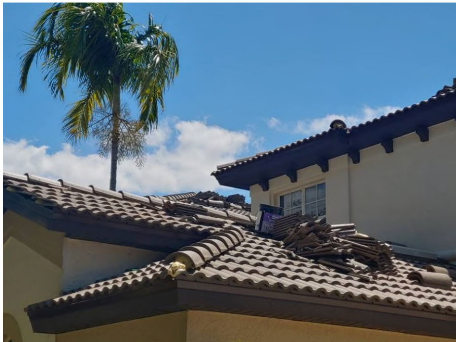
Photograph #2: Roof field, ridge and hip tile installations with polyurethane foam adhesive were in progress on building 21710.
