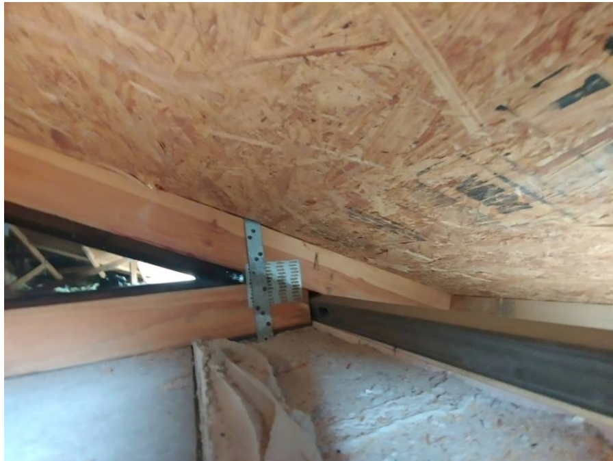
Photograph #22: Existing strap clips on trusses have the required minimum quantity of nails on building 21731. Installation of new hurricane truss anchor straps (HGAM10) is not required.
