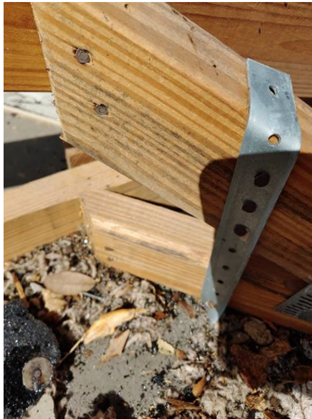
Photograph #5: KEG observed a lack of nails on a few existing straps on building 7861. N8D nails were installed during the site visit to comply with the Florida building code.
