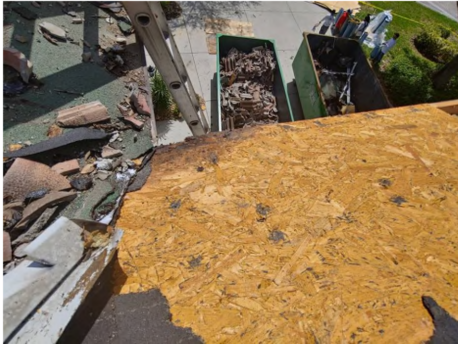
Photograph #3: Rotten plywood sheathing was observed on building 7861.
