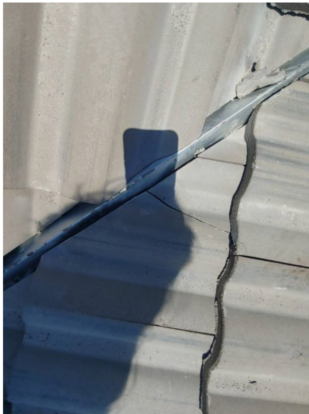
Photograph #12: Broken field tile replacement must be addressed on building 21721.
