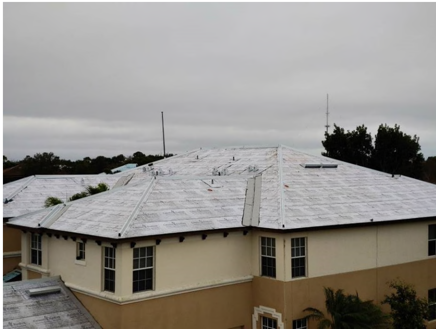
Photograph #9: V-crimp metal valley flashing, and hip/ridge metal channel installations were in progress on building 21710.
