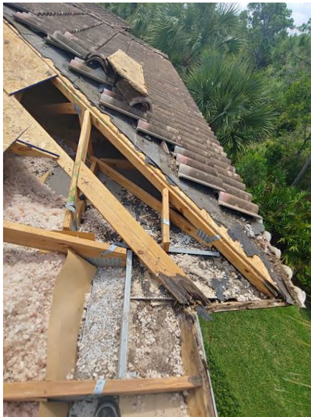
Photograph #28: Rotten fascia and truss were observed on building 21820.
