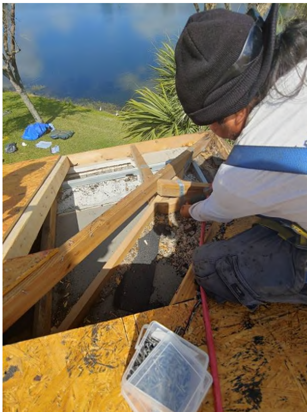
Photograph #6: KEG observed a lack of nails on a few existing straps on building 7861. N8D nails were installed during the site visit to comply with the Florida building code.
