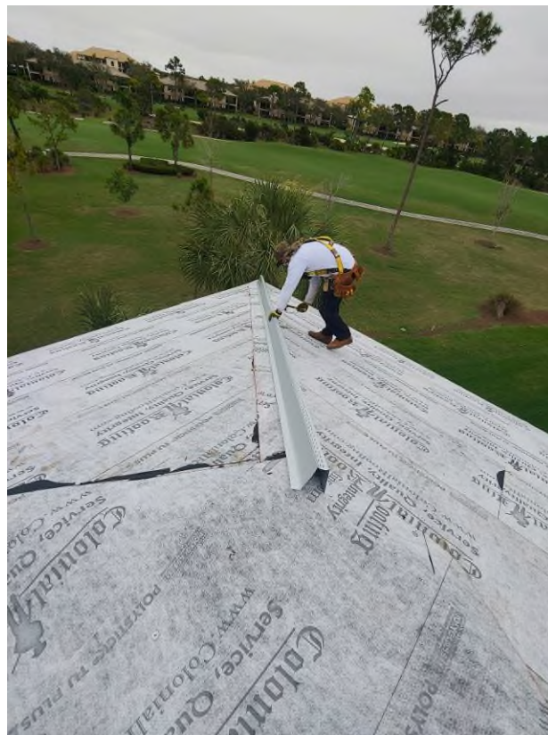
Photograph #12: V-crimp metal valley flashing, and hip/ridge metal channel installations were in progress on building 21711.
