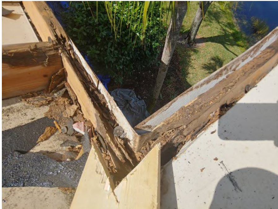
Photograph #2: Rotten wood fascia was observed on building 7861.
