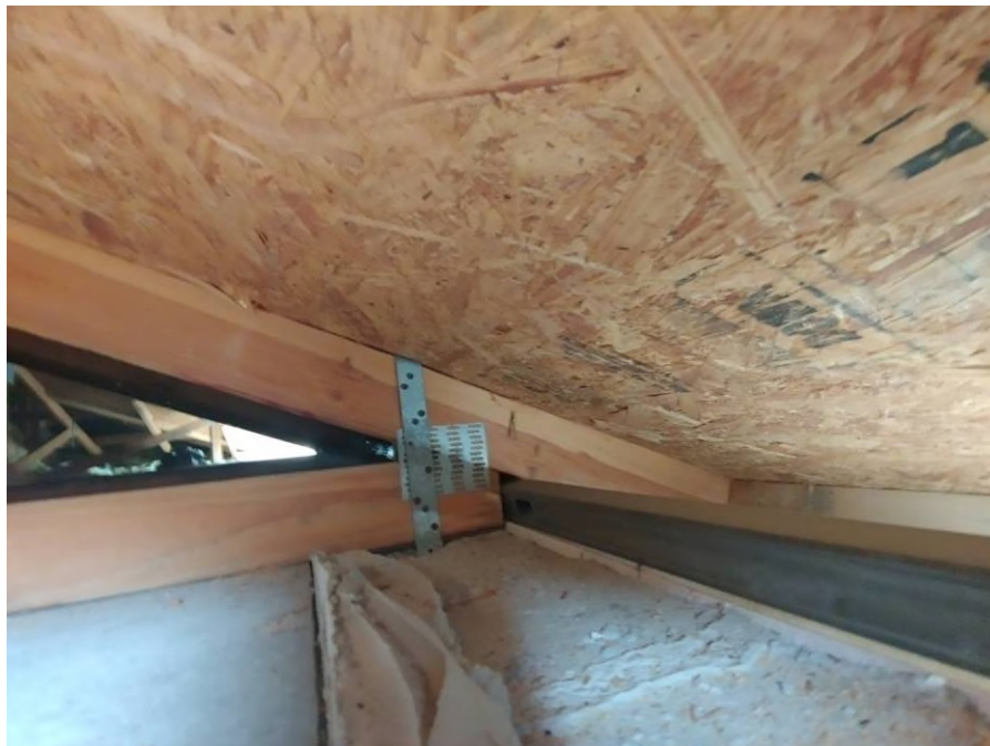
Photograph #22: Existing strap clips on trusses have the required minimum quantity of nails on building 21731. Installation of new hurricane truss anchor straps (HGAM10) is not required.
