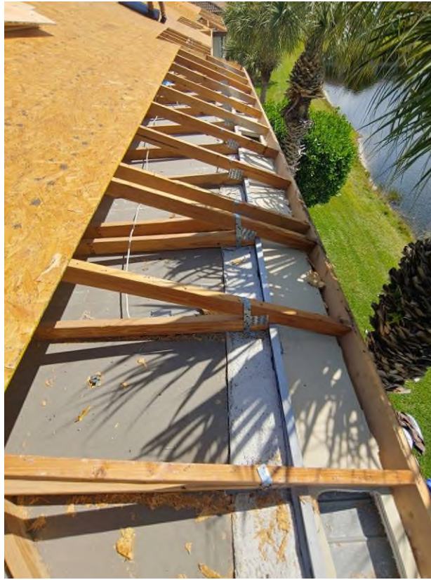
Photograph #11: Existing strap clips on the trusses have the required minimum quantity of nails on building 21750.
