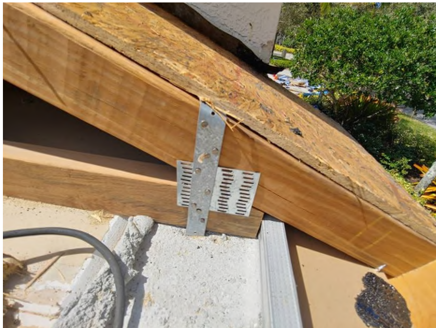
Photograph #8: Existing strap clips on the trusses have the required minimum quantity of nails on building 21740
