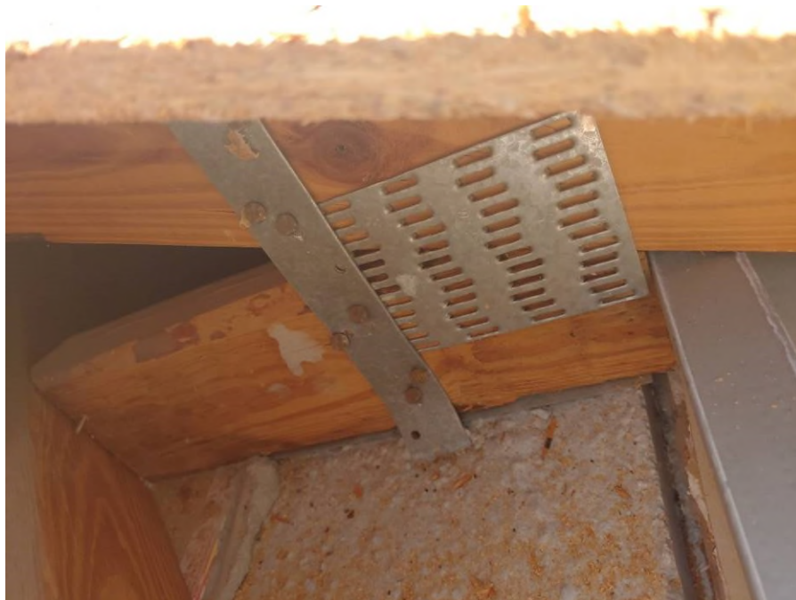
Photograph #2: Existing strap clips on the trusses have the required minimum quantity of nails on building 7870.
