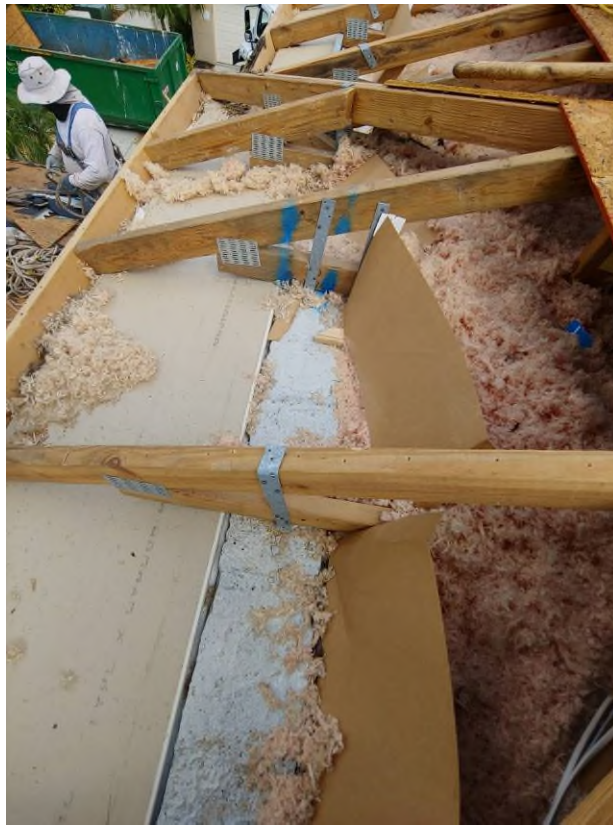
Photograph #1: Existing strap clips on the trusses have the required minimum quantity of nails on building 7870.
