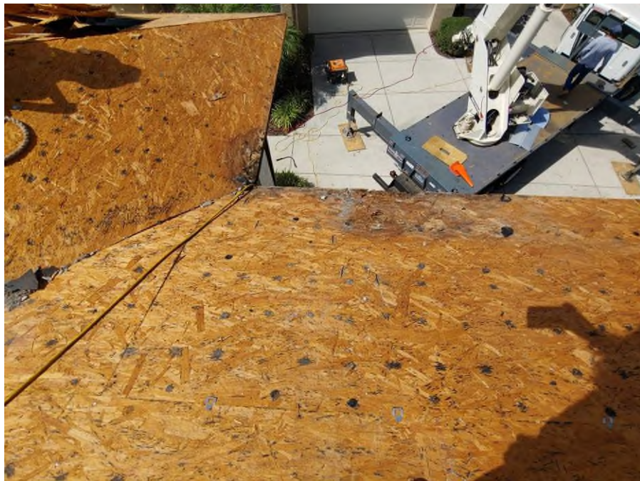
Photograph #14: Rotten plywood sheathing was observed on building 21750.
