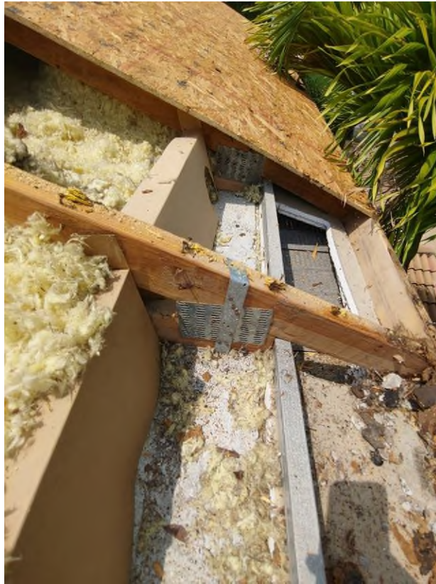
Photograph #9: Existing strap clips on the trusses have the required minimum quantity of 5 nails on building 21801.
