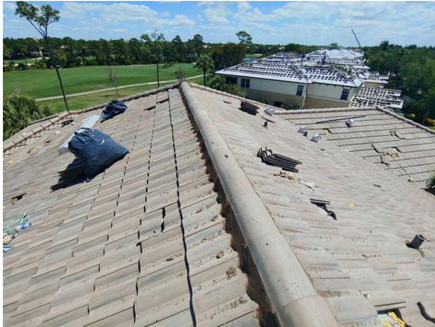
Photograph #5: Roof field, ridge and hip tile installations with polyurethane foam adhesive were in progress on building 21711.
