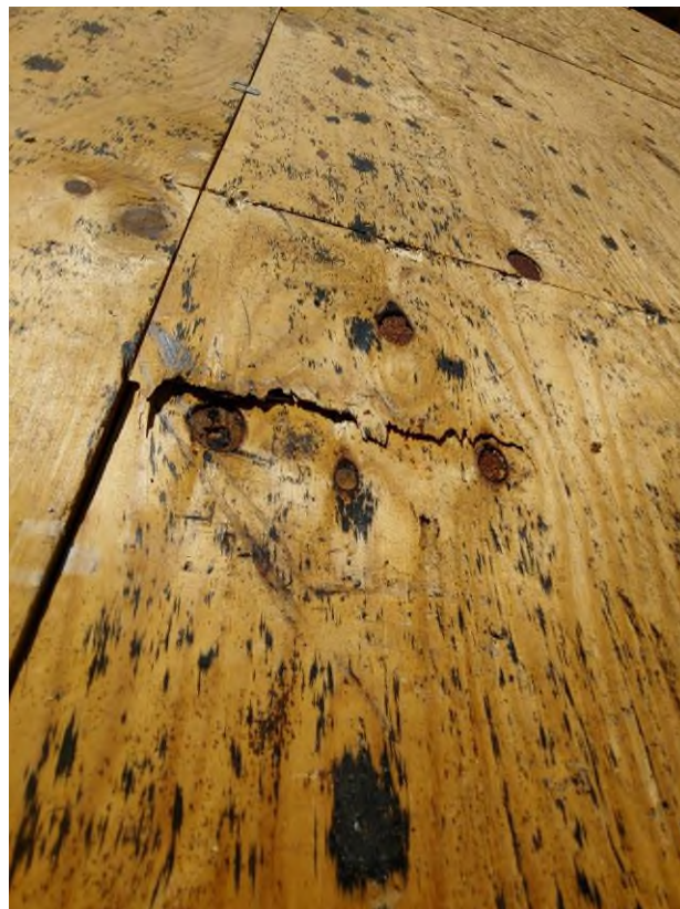
Photograph #16: Broken plywood sheathing was observed on building 21810. Contractor must replace.
