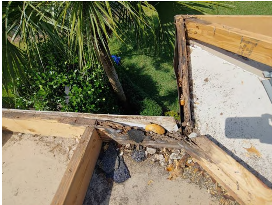
Photograph #15: Rotten fascia and truss were observed on building 21810.
