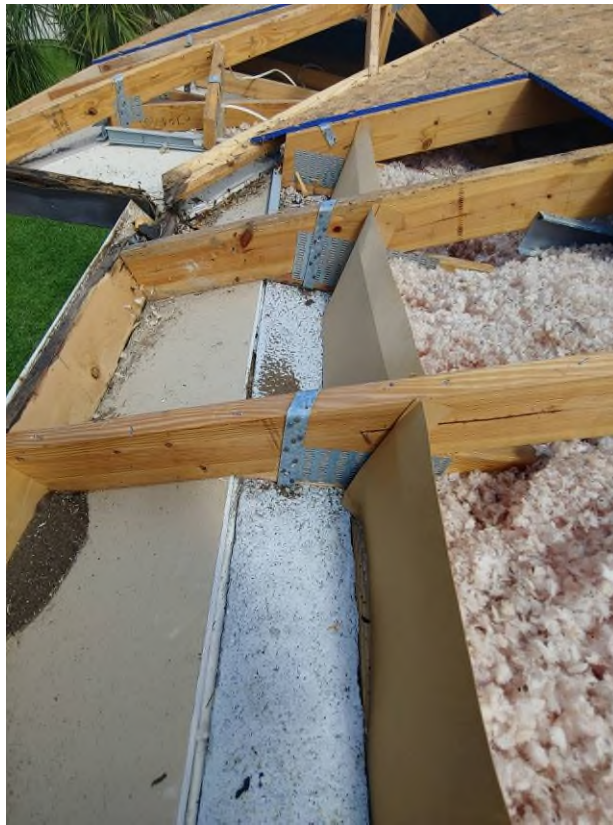
Photograph #13: Existing strap clips on the trusses have the required minimum of nails on building 21810.
