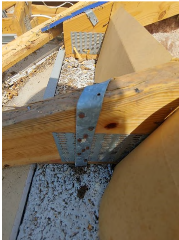
Photograph #14: Existing strap clips on the trusses have the required minimum of nails on building 21810.
