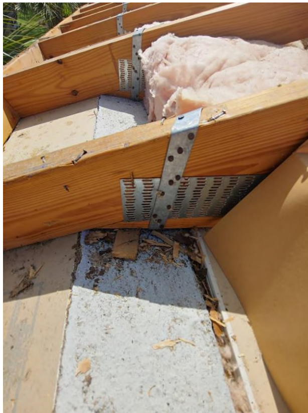
Photograph #8: Existing strap clips on the trusses have the required minimum of nails on building 21771.
