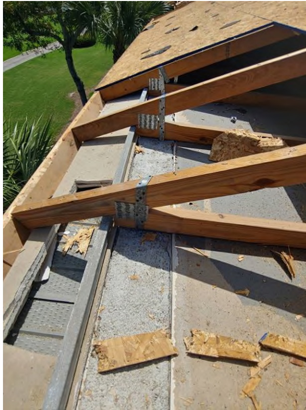
Photograph #7: Existing strap clips on the trusses have the required minimum of nails on building 21771.
