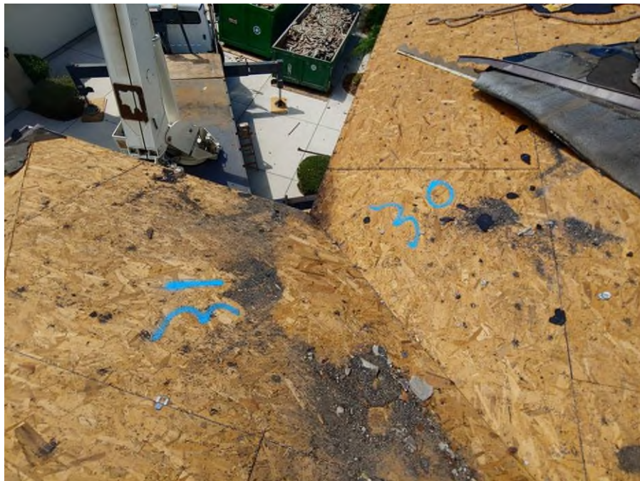
Photograph #10: Rotten plywood sheathing was observed on building 21771.
