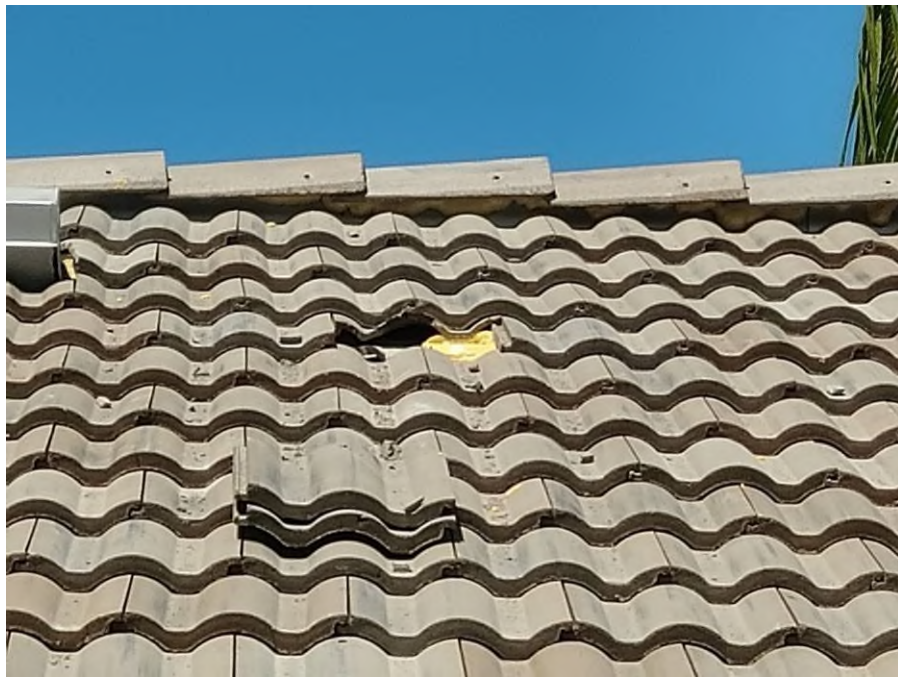
Photograph #4: Broken field tile replacement must be addressed on building 21710.
