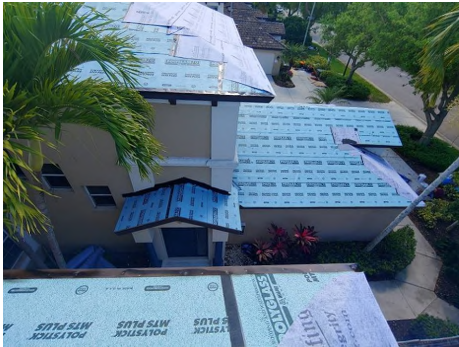
Photograph #5: Drip-edge installation was in progress on the garage roof of building 21761.
