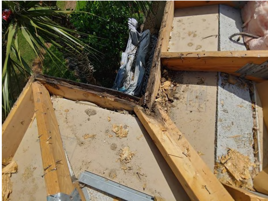
Photograph #9: Rotten fascia and truss were observed on building 21771.
