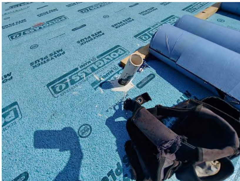
Photograph #4: Sealant application surrounding the exhaust vent pipe was in progress on building 21840.
