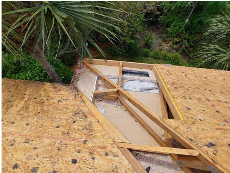
Photograph #8: Rotten fascia, truss and plywood sheathing were observed on building 21850.
