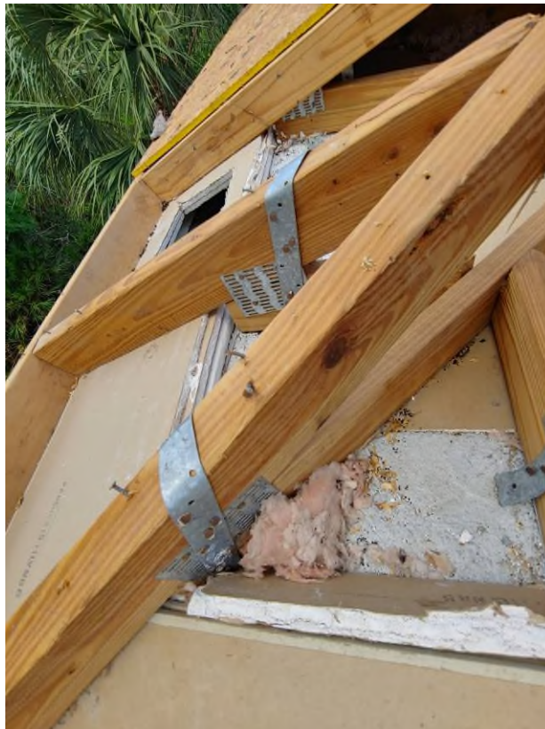
Photograph #6: Existing strap clips on the trusses have the required minimum quantity of 5 nails on building 21850.
