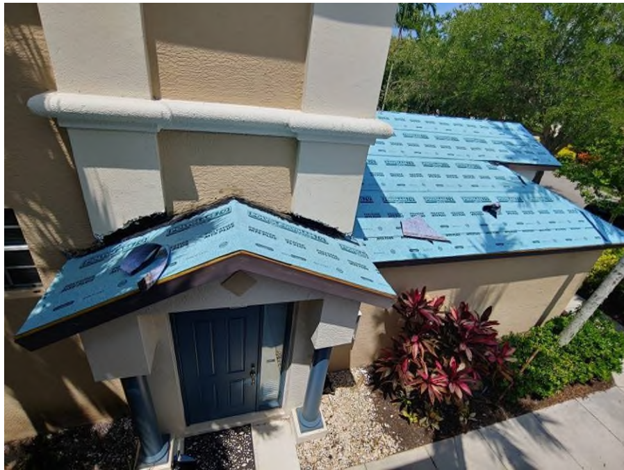
Photograph #3: Missing drip-edge flashing installation was observed on the garage of building 21840.
