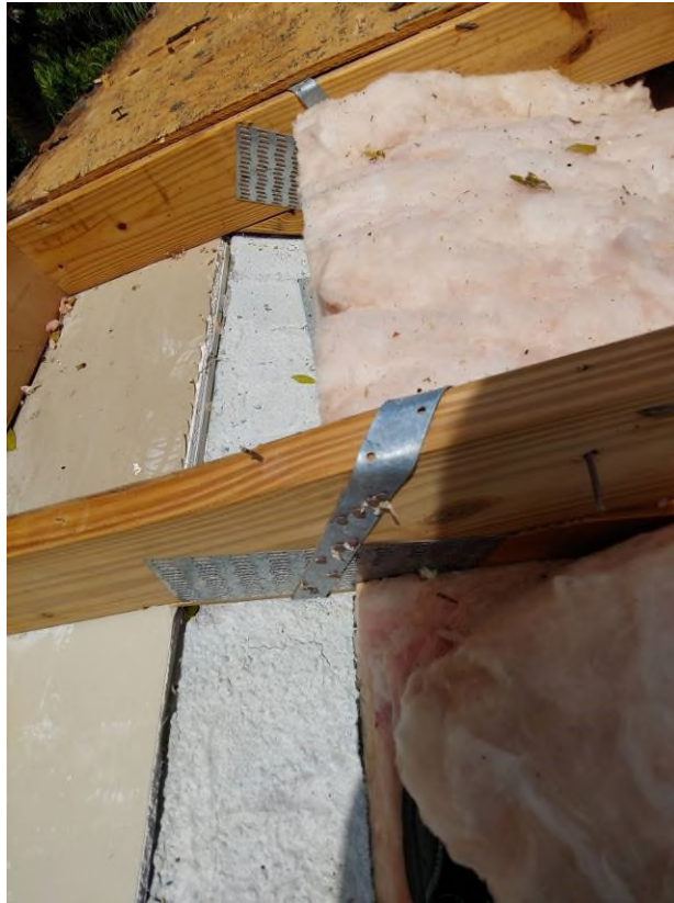
Photograph #7: Existing strap clips on the trusses have the required minimum quantity of 5 nails on building 21850.
