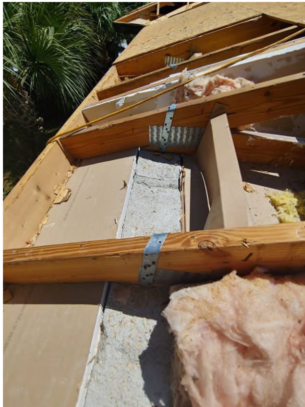
Photograph #12: Existing strap clips on the trusses have the required minimum of 5 nails on building 21841.
