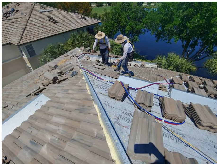
Photograph #4: Roof field, ridge and hip tile installations with polyurethane foam adhesive were in progress on building 7861.
