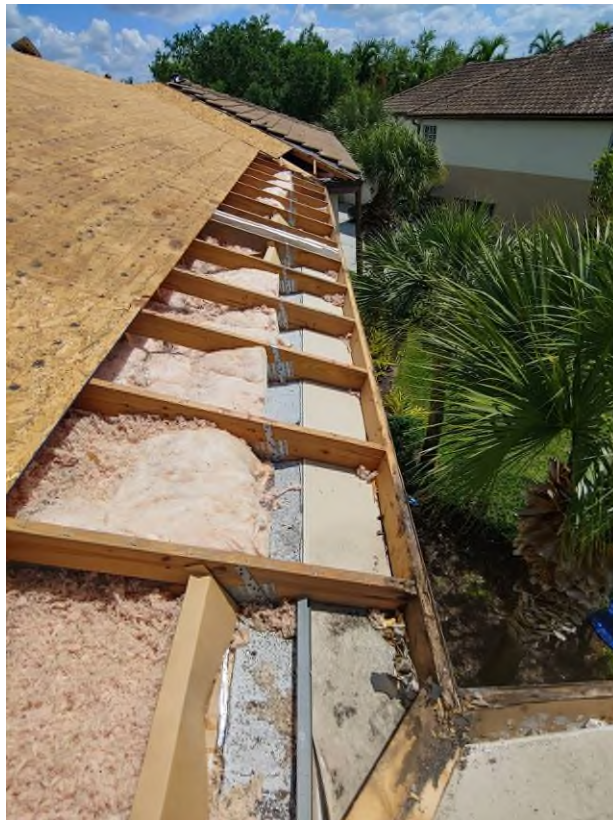
Photograph #12: Existing strap clips on the trusses have the required minimum of nails on building 21800.
