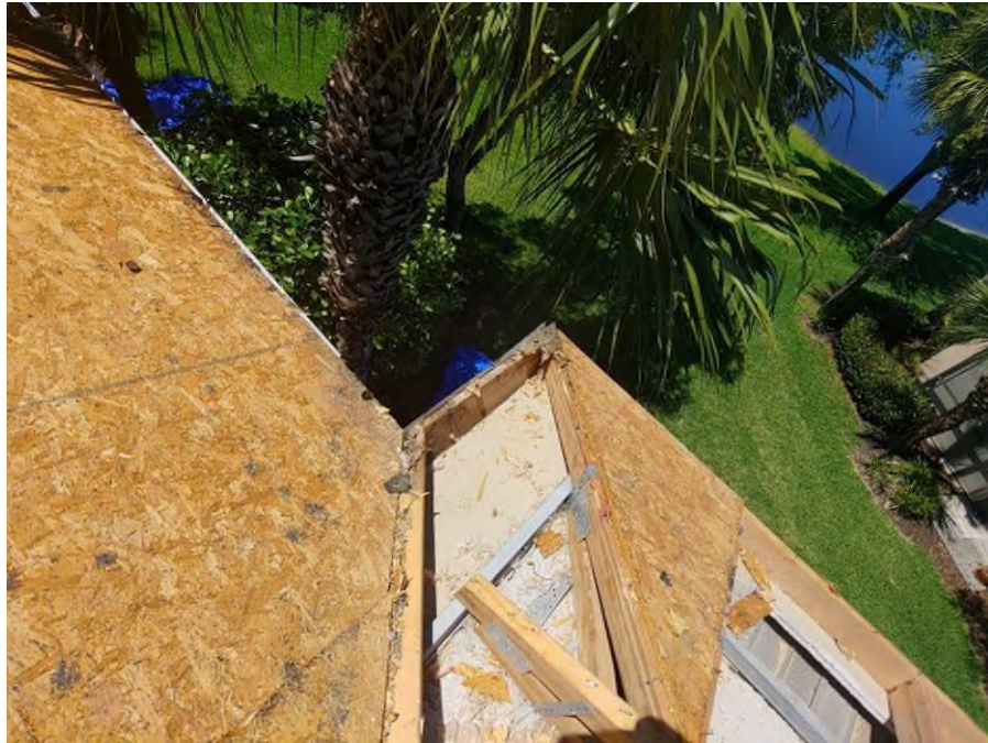
Photograph #11: Rotten fascia, truss and plywood sheathing were observed and marked for replacement on building 21780.
