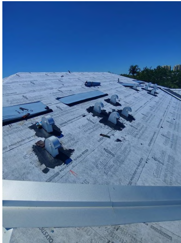
Photograph #13: Asphalt plastic roofing cement application surrounding the exhaust vents and v-crimp metal valley flashing was in progress on building 21800.
