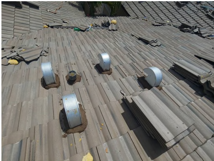
Photograph #4: Mortar adhesive application was in progress surrounding the exhaust vents and pipes on building 21700.
