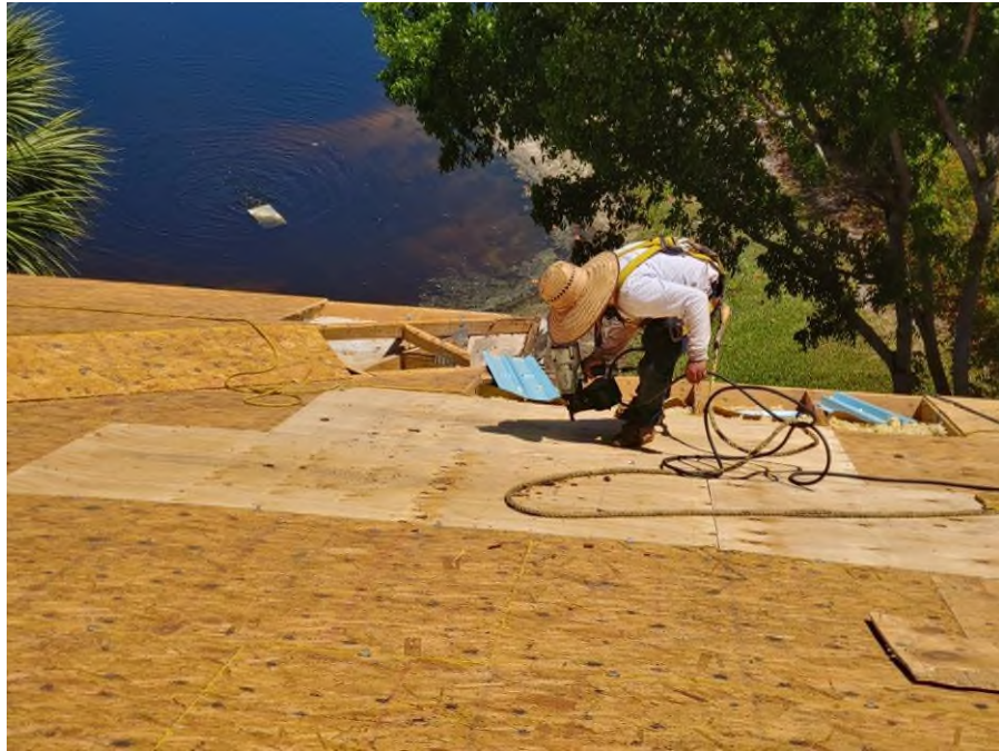
Photograph #9: Re-nail pattern at the plywood sheathing was in progress on building 21831.
