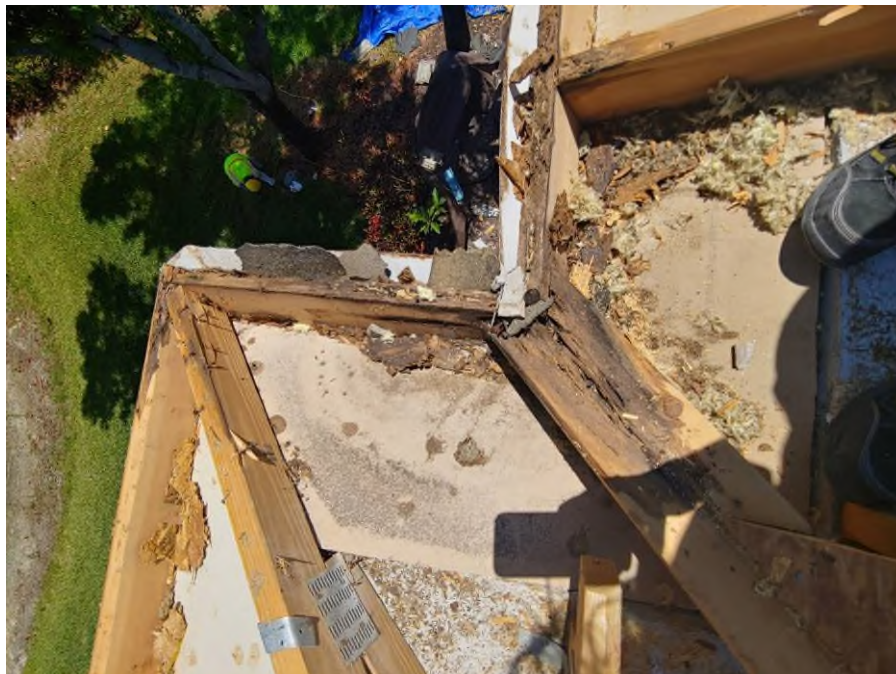
Photograph #8: Rotten fascia and truss were observed on building 21831.
