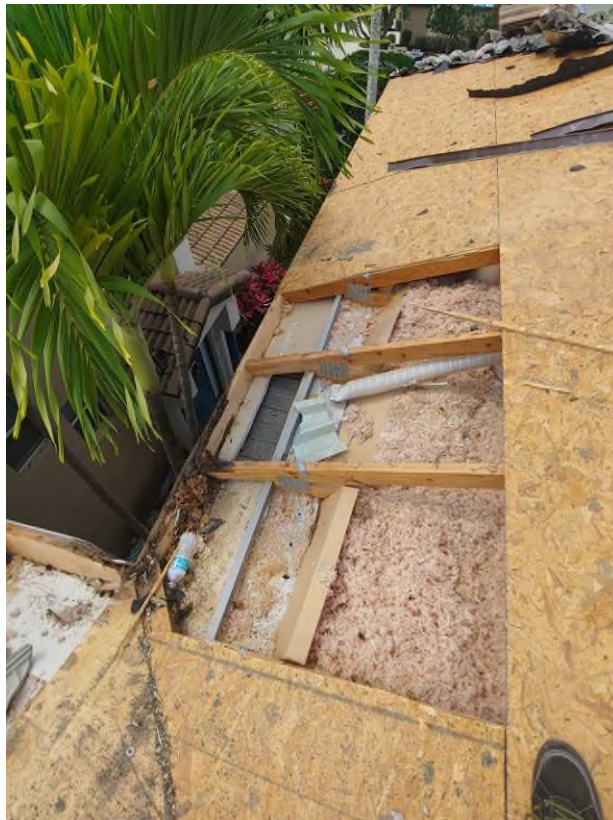
Photograph #10: Existing strap clips on the trusses have the required minimum quantity of nails on building 21771.
