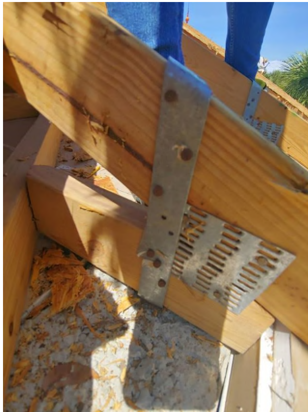
Photograph #6: Existing strap clips on the trusses have the required minimum of 5 nails on building 21831.
