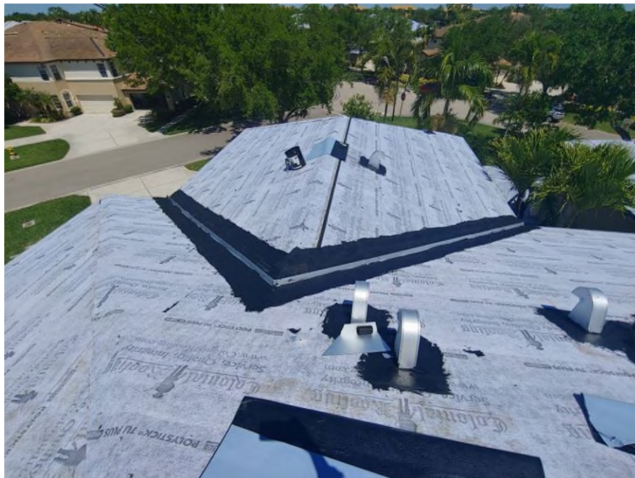
Photograph #14: Asphalt plastic roofing cement application surrounding the exhaust vents and v-crimp metal valley flashing was in progress on building 21800.
