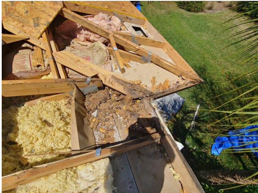
Photograph #14: Rotten fascia and truss were observed on building 21841.
