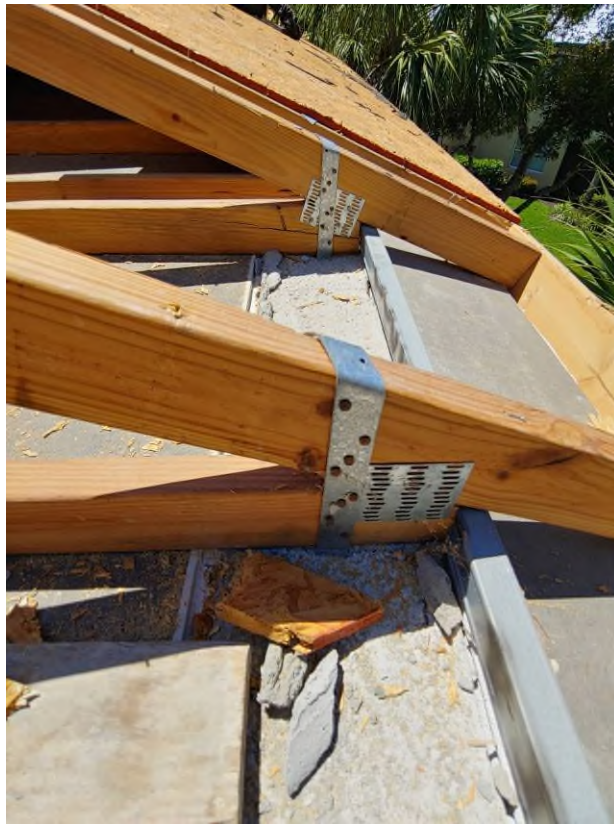
Photograph #9: Existing strap clips on the trusses have the required minimum of 5 nails on building 21780.
