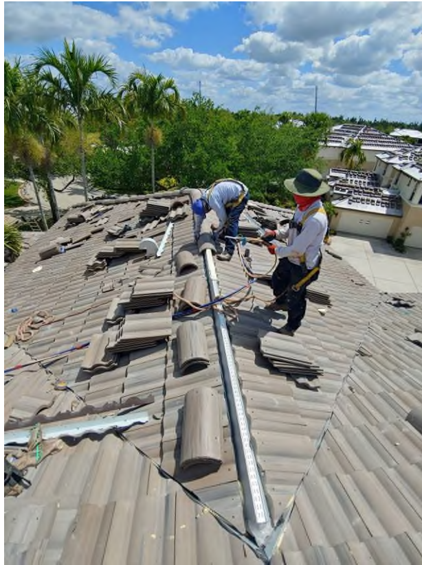
Photograph #3: Roof field, ridge and hip tile installations with polyurethane foam adhesive were in progress on building 21700.
