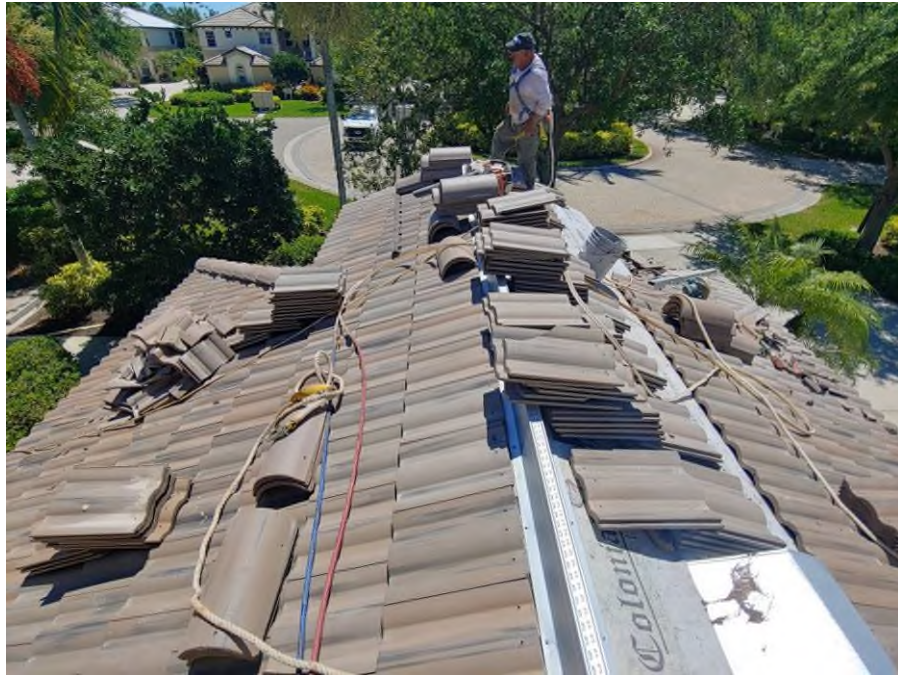
Photograph #1: Roof field, ridge and hip tile installations with polyurethane foam adhesive were in progress on building 7851.
