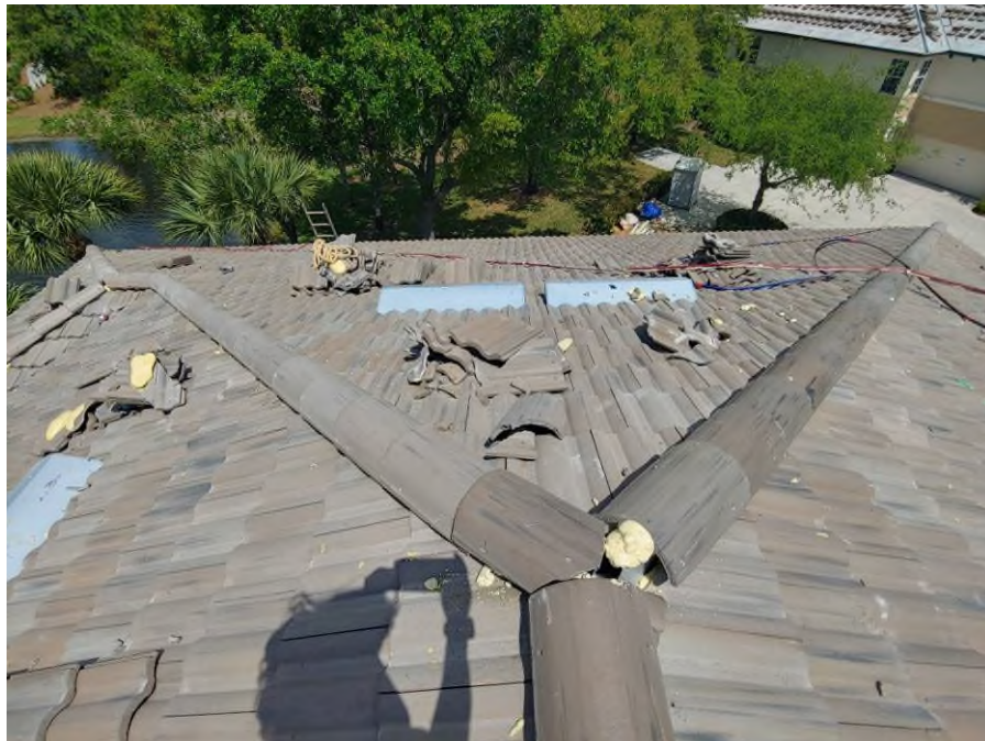
Photograph #2: Roof field, ridge and hip tile installations with polyurethane foam adhesive were in progress on building 21700.
