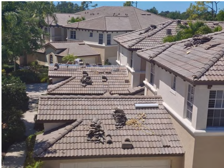
Photograph #2: Roof field, ridge and hip tile installations with polyurethane foam adhesive were in progress on building 7851.
