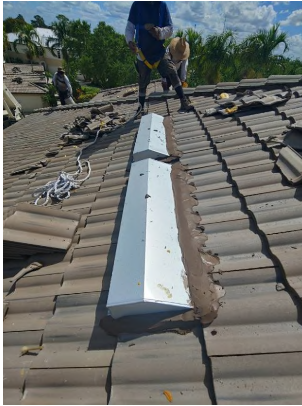
Photograph #3: Mortar adhesive application was in progress surrounding the exhaust vents on building 21700.
