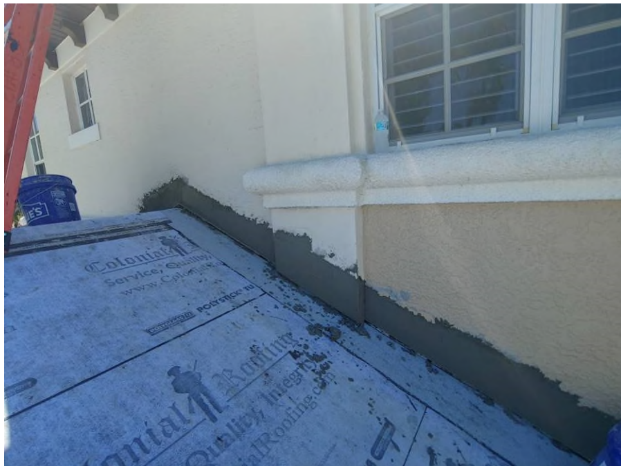
Photograph #12: Stucco application was in progress at the bottom of the wall and columns on building 21800.
