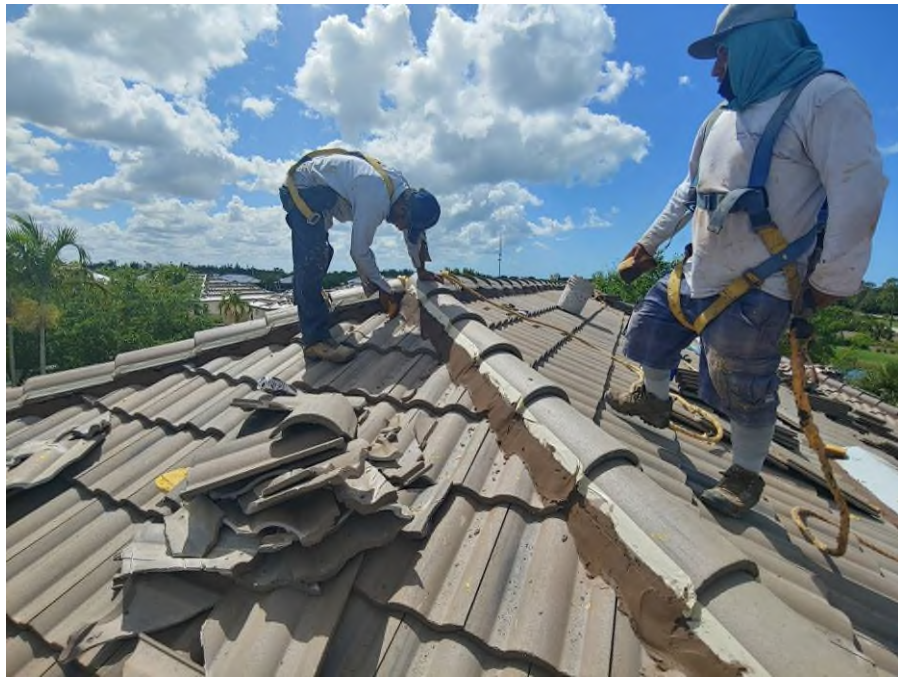
Photograph #5: Mortar adhesive application was in progress surrounding the hip and ridge tiles on building 21700.
