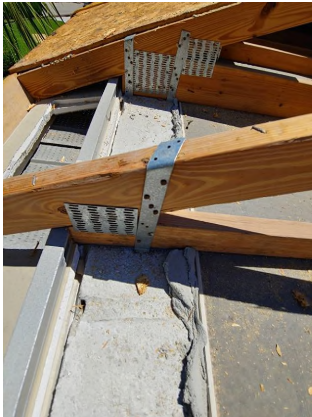
Photograph #8: Existing strap clips on the trusses have the required minimum of 5 nails on building 21780.
