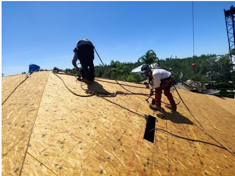
Photograph #15: Re-nail pattern at the plywood sheathing was in progress on building 21841.
