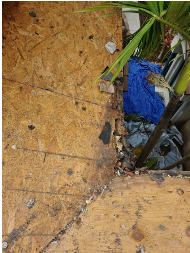
Photograph #12: Rotten fascia, truss and plywood sheathing were observed on building 21771.
