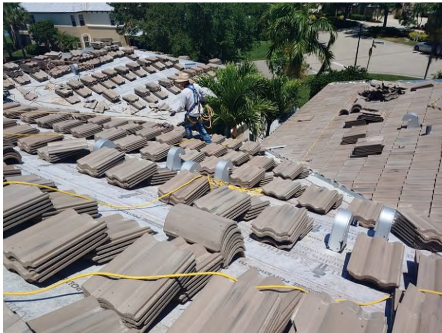
Photograph #2: Roof field tile installation with polyurethane foam adhesive was in progress on building 21800.
