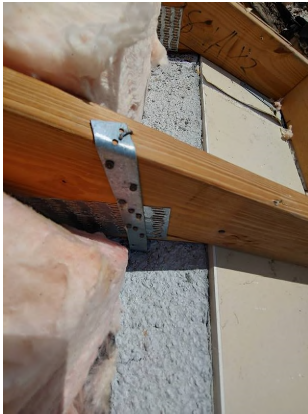
Photograph #13: Existing strap clips on the trusses have the required minimum of nails on building 21800.
