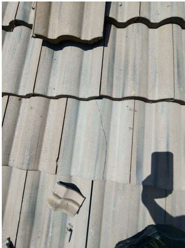
Photograph #4: Contractor must replace the broken-field tiles that were noted on building 21700 during the site visit.
