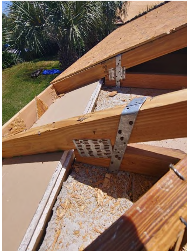
Photograph #7: Existing strap clips on the trusses have the required minimum of 5 nails on building 21831.
