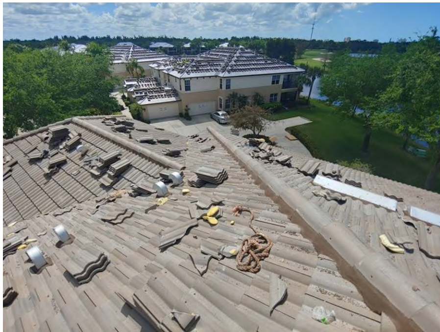
Photograph #6: Mortar adhesive application was in progress surrounding the hip and ridge tiles on building 21700.
