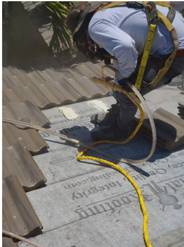
Photograph #5: Roof field, ridge and hip tile installations with polyurethane foam adhesive were in progress on building 7861.
