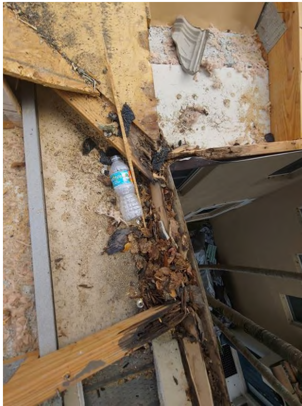
Photograph #13: Rotten fascia, truss and plywood sheathing were observed on building 21771.
