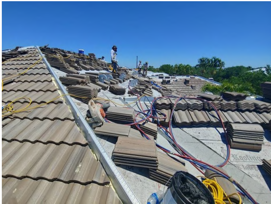
Photograph #3: Roof field, ridge and hip tile installations with polyurethane foam adhesive were in progress on building 7861.
