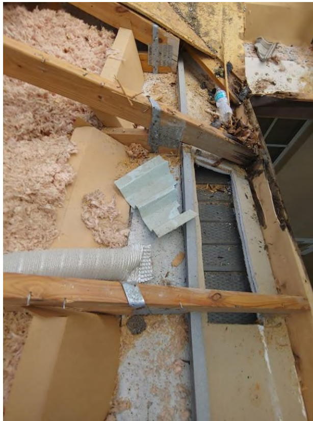
Photograph #11: Existing strap clips on the trusses have the required minimum quantity of nails on building 21771.
