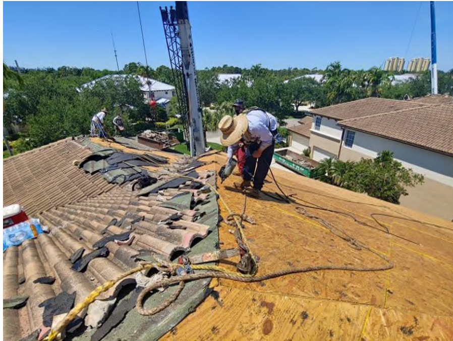
Photograph #11: Re-nail pattern at the plywood sheathing was in progress on building 21841.
