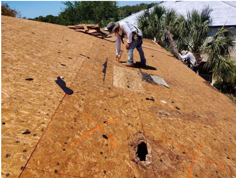
Photograph #10: Rotten fascia, truss and plywood sheathing were observed and marked for replacement on building 21780.
