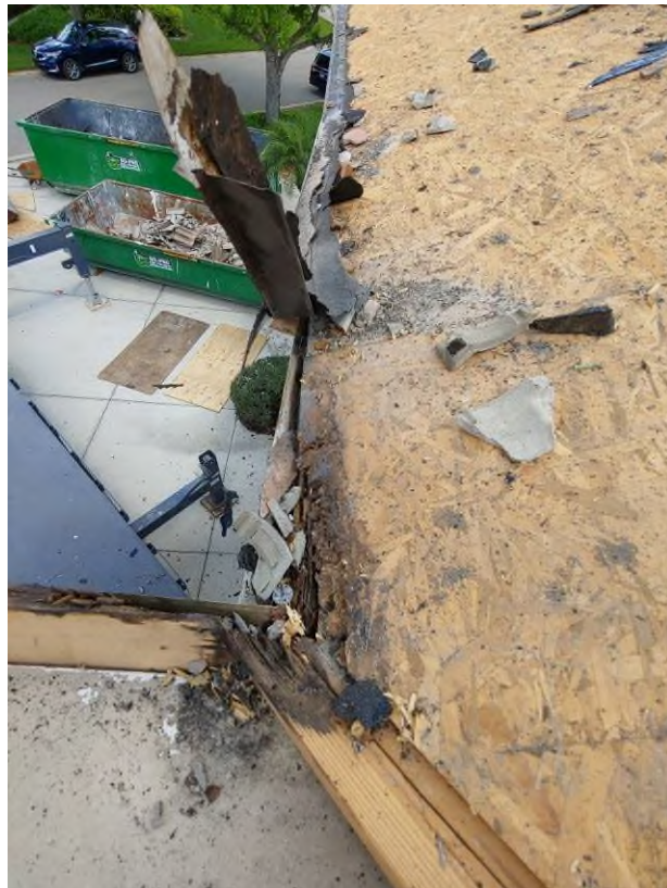
Photograph #14: Rotten fascia, truss and plywood sheathing were observed on building 21800.
