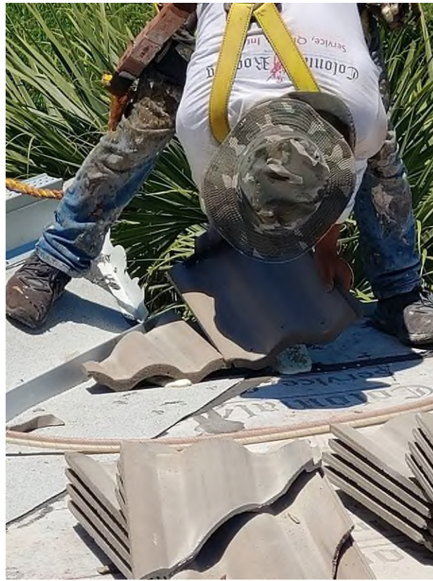
Photograph #3: Roof field tile installation with polyurethane foam adhesive was in progress on building 21800.
