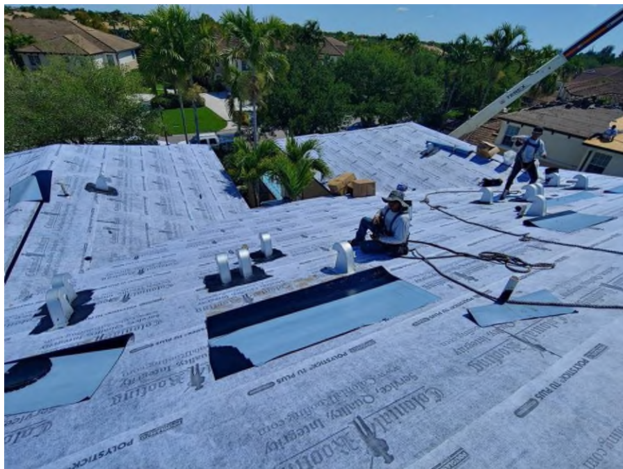
Photograph #4: Asphalt plastic roofing cement application was in progress surrounding the exhaust vents on building 21820.
