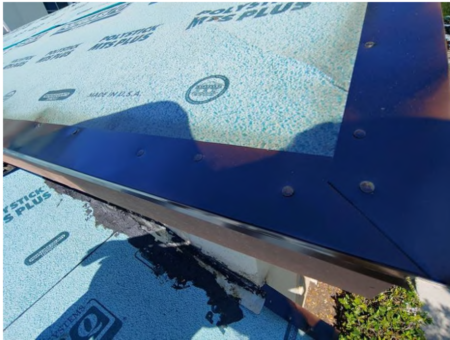
Photograph #5: Drip-edge flashing installation was in progress on the garage roof on building 21820.
