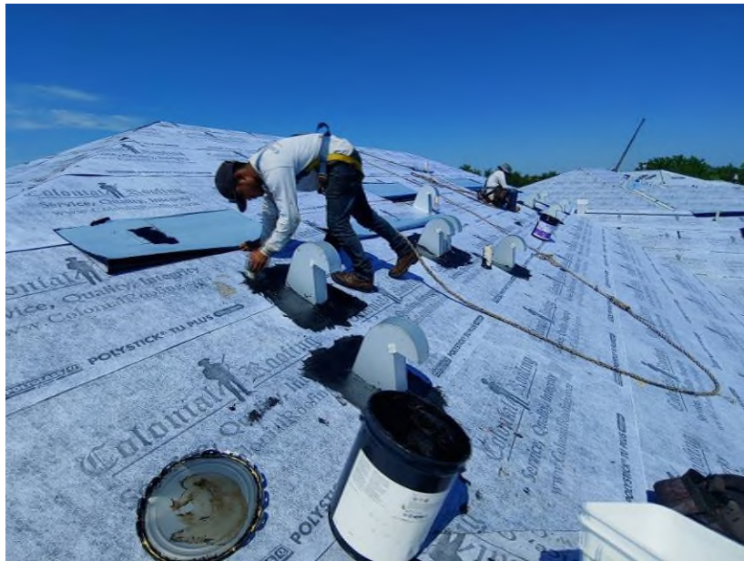
Photograph #3: Asphalt plastic roofing cement application was in progress surrounding the exhaust vents on building 21820.
