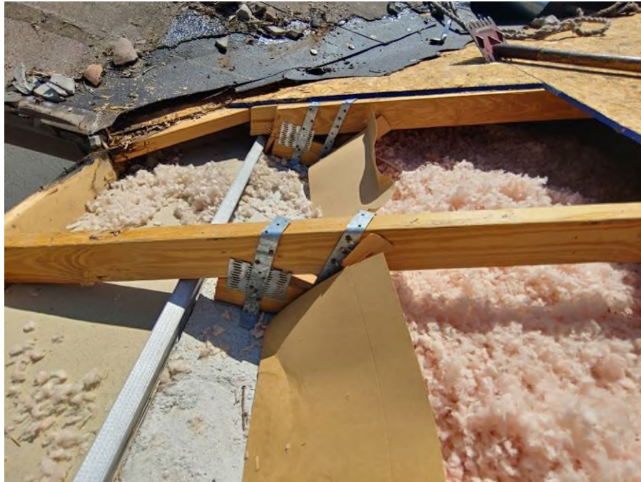
Photograph #9: Existing strap clips on the trusses have the required minimum quantity of 5 nails on building 21830.
