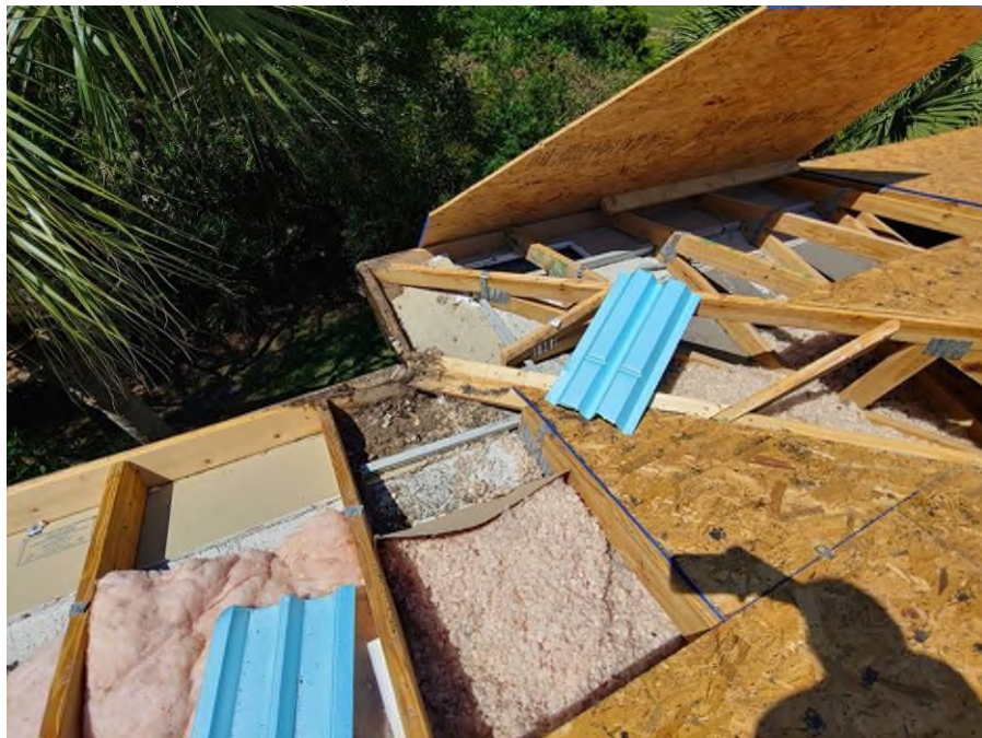
Photograph #10: Rotten fascia, truss and plywood sheathing were observed on building 21830.
