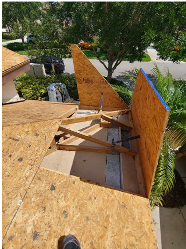
Photograph #8: Existing strap clips on the trusses have the required minimum of 5 nails on building 21830.
