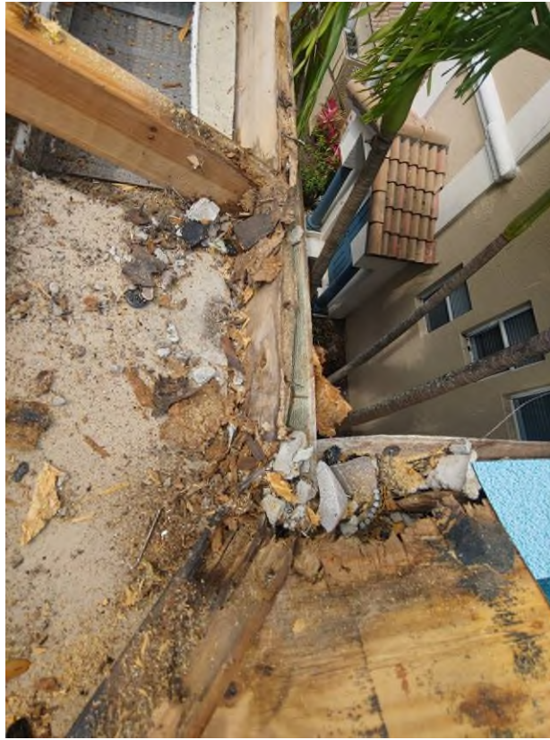
Photograph #11: Rotten fascia, trusses and plywood sheathing were observed on building 21801.
