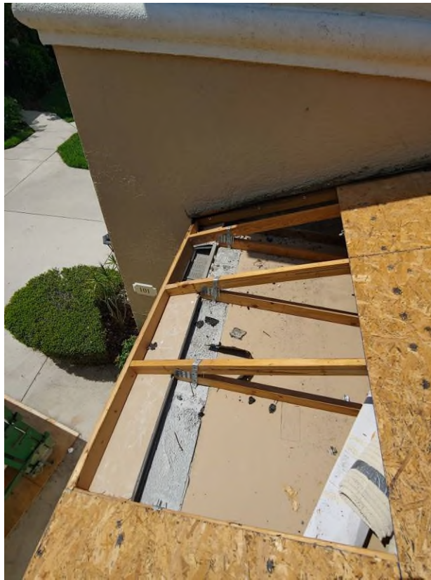
Photograph #7: Existing strap clips on the trusses have the required minimum of 5 nails on building 21830.
