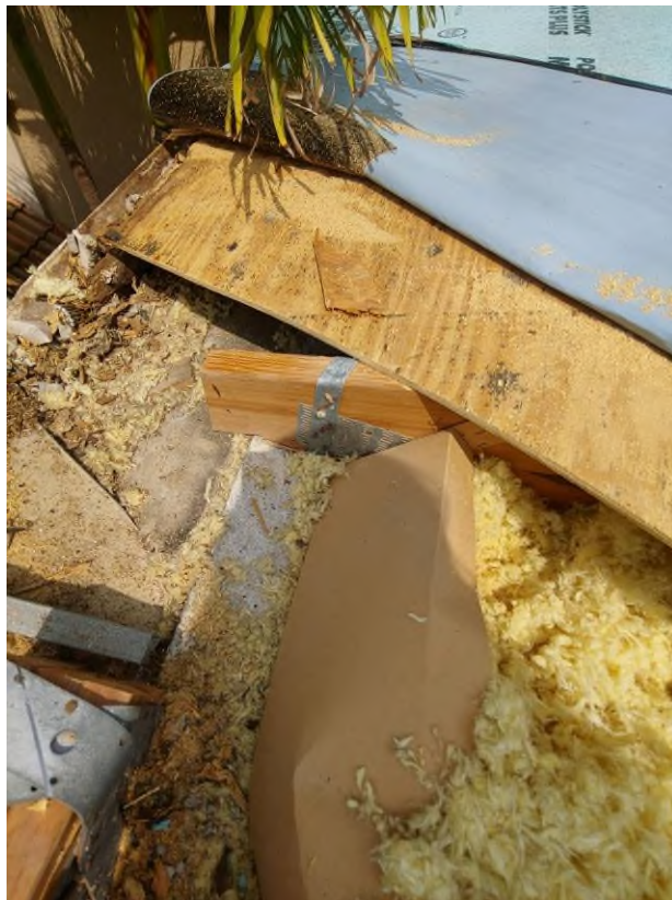
Photograph #10: Existing strap clips on the trusses have the required minimum quantity of 5 nails on building 21801.
