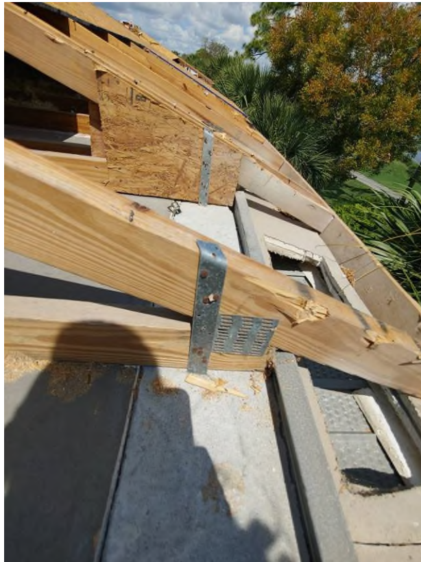
Photograph #4: Existing strap clips on the trusses have the required minimum of 5 nails on building 21791.
