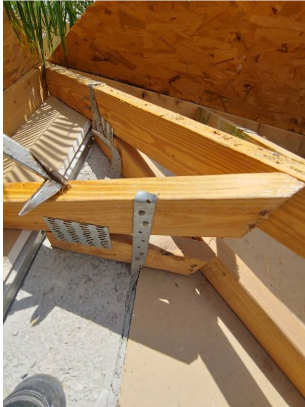
Photograph #9: Existing strap clips on the trusses have the required minimum of 5 nails on building 21830.
