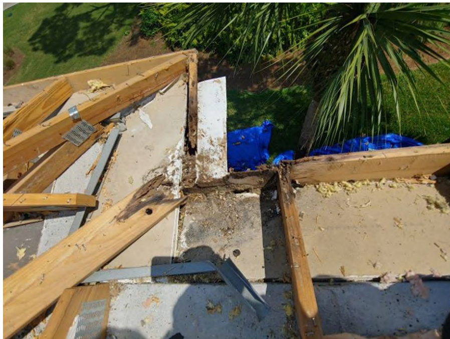
Photograph #6: Rotten fascia, truss and plywood sheathing were observed on building 21791.
