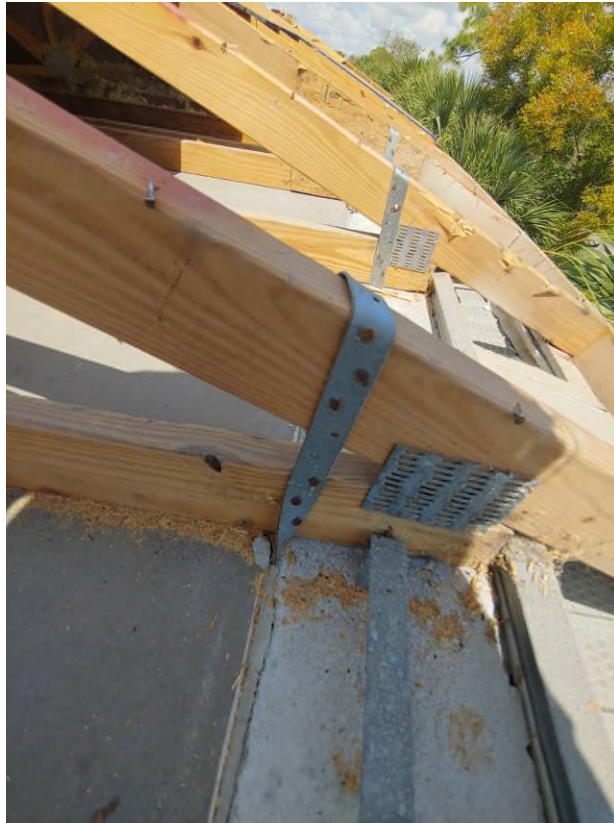
Photograph #3: Existing strap clips on the trusses have the required minimum of 5 nails on building 21791.
