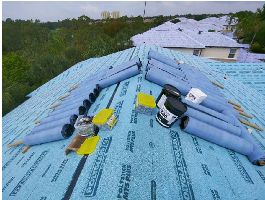
Photograph #5: Second layer of underlayment installation was set in place for installation on building 21840.
