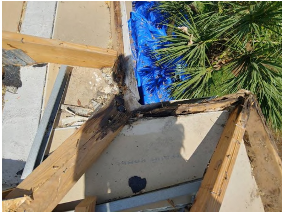
Photograph #5: Rotten fascia, truss and plywood sheathing were observed on building 21791.
