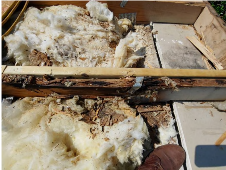
Photograph #15: Rotten fascia, trusses and plywood sheathing were observed on building 21811.
