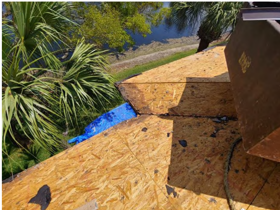
Photograph #16: Rotten fascia, trusses and plywood sheathing were observed on building 21811.
