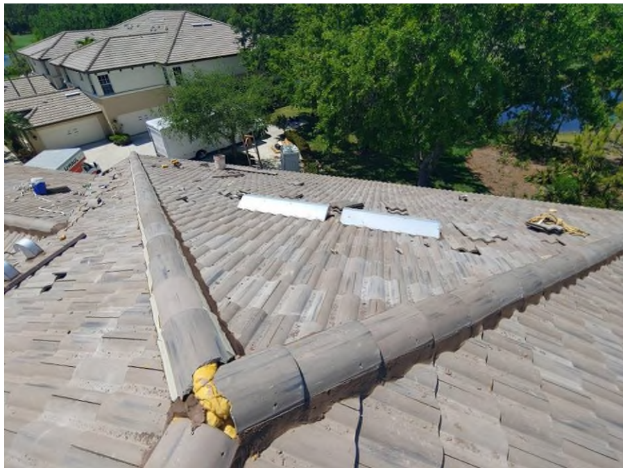
Photograph #6: Roof field, ridge and hip tile installations with polyurethane foam adhesive were in progress on building 21711.
